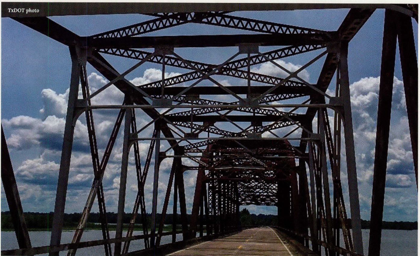
The truss on the Neches River Bridge after critical repairs were completed.
