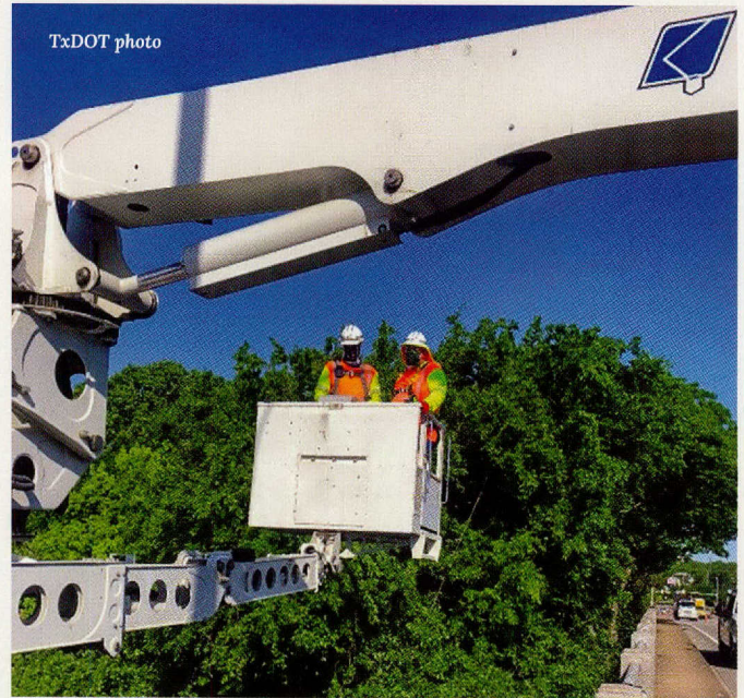
Josh Gutzwiller (left) and John Henry are wearing face masks while inspecting a damaged bridge in the Beaumont District.
