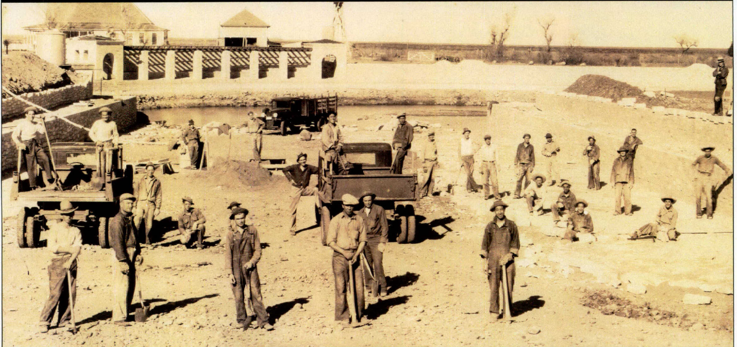
Civilian Conservation Corps workers build the swimming pool at Balmorhea State Park.
