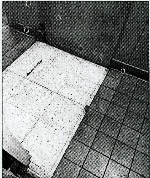
FIGURE 9-7 GONZALES ISD HIGH SCHOOL KITCHEN FLOORING MARCH 2020
