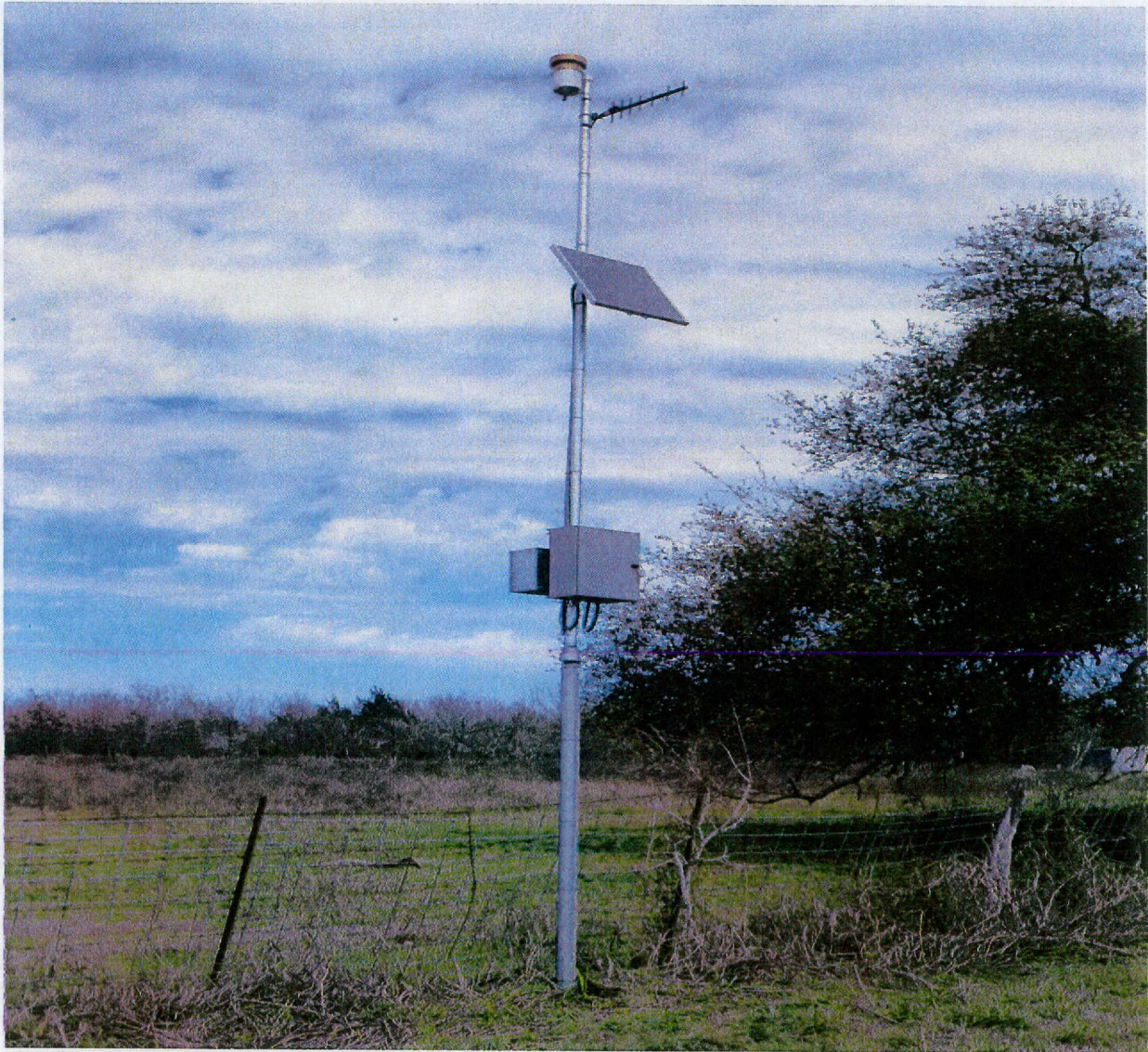
FIGURE "B-6" Rain Gauges Installed
