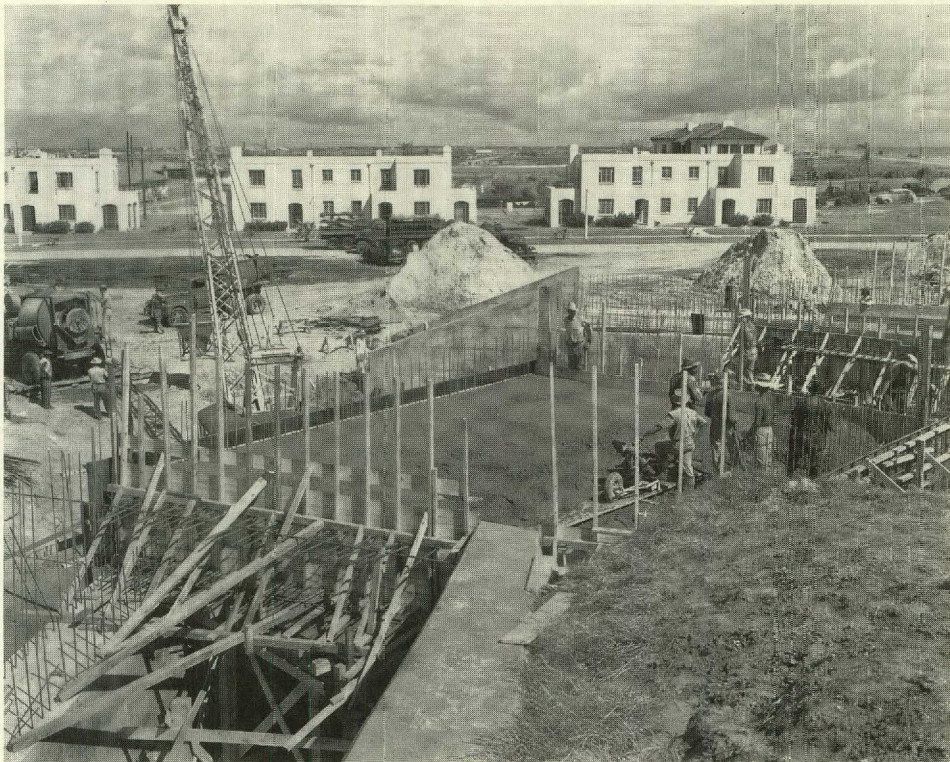
Corps of Engineers workmen pouring concrete at Battery Hoskins, Fort Crockett, 1942. Photo courtesy of U.S. Army Corps of Engineers archives, Galveston, Texas.
