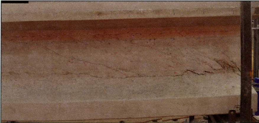
Tx46-II (West side)
