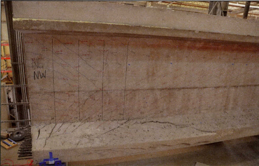
Tx70-II (West side)
