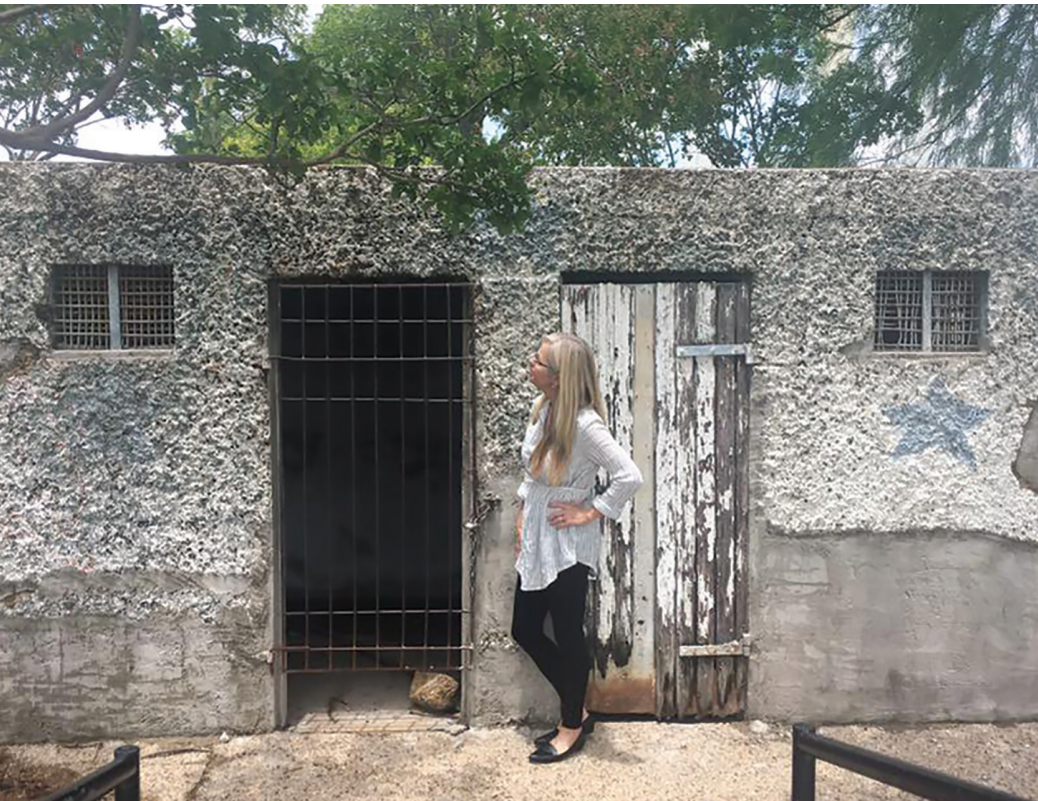
Top: Large cracks in the calaboose threatened the building's structural integrity and signaled its impending collapse. Photograph courtesy of William E. Moore. Bottom: Royse City Chamber of Commerce official Julia Bryant, now retired, was a key player in the restoration of the historic structure. Image provided by the Royse City Chamber of Commerce.
