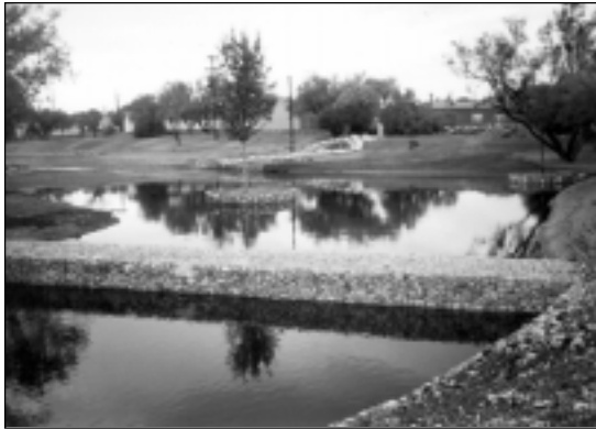
This structure, designed to detain and filter urban runoff, was constructed at Santa Rita Park in San Angelo.
