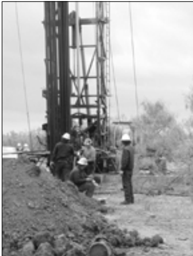
A contractor pumps a cement plug into an unplugged oil well in Mitchell County.
