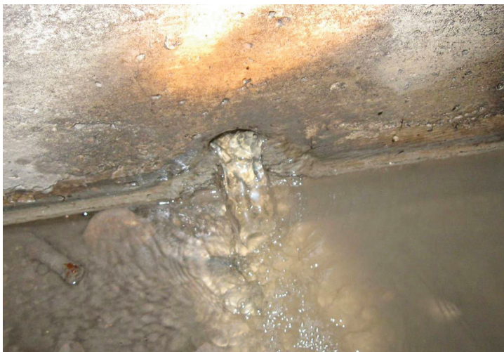
Weep hole in sanitary sewer main (photo courtesy of SAWS)
