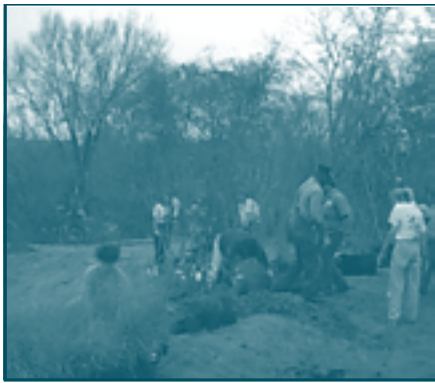
Members of Keep Smithville Beautiful, the garden club, city workers and officials, and LCRA staff participated in landscaping the project. Many of the plants were donated.
