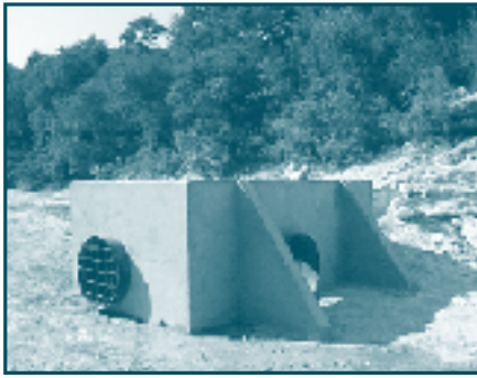
Antioch Cave BMP on Onion Creek during dry conditions. The 26-inch valve in the end of the concrete vault is protected by a welded steel grill. A blanked-off flange for clean-out needs or possible future installation of a second valve can be seen on the side between the buttresses. The BMP is about 6 feet high, 7 feet wide, and 13 feet long.
