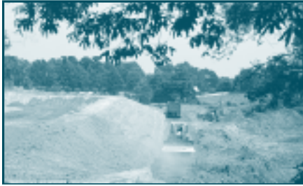
The Chireno ISD discharge system in Nacogdoches County handles 10,000 gallons per day with three clay lined cells. The system was placed on a steep slope with two cells up-slope and a large third cell shown here under construction.
