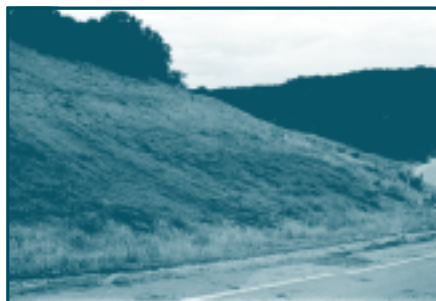
Oasis Bluff Drive site after restoration. A total of 6.26 acres of roadside were revegetated under this project.
