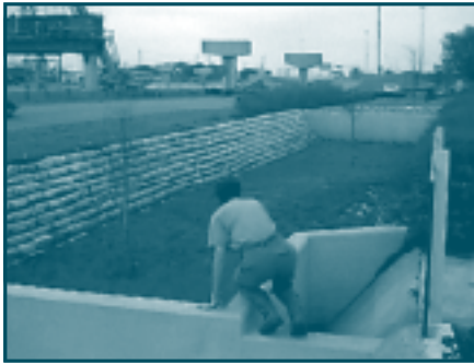
Inspectors ensure that BMP structures in the Edwards Aquifer recharge zone are properly maintained so that they continue to be effective in reducing pollutant loads.
