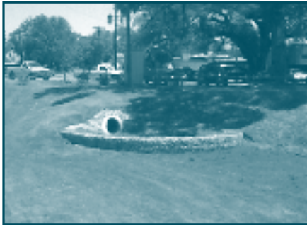
The first stage of the Smithville BMP is an extended detention pond with underground filtration chambers.
