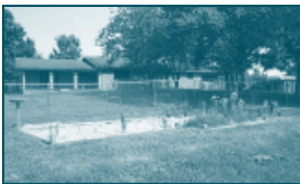
Finished single family on-site system. Wetlands and drainfield are located below the house.
