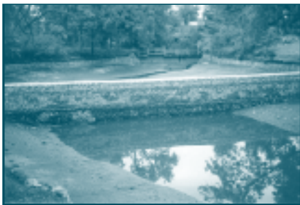
The structural BMP at Civic League Park rock gabion berm and retention pond.
