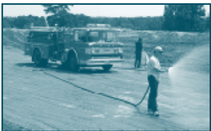
The clay liner had to meet compaction and moisture specifications. The local fire department assisted the contractor with hauling and spraying water to meet the moisture requirement.
