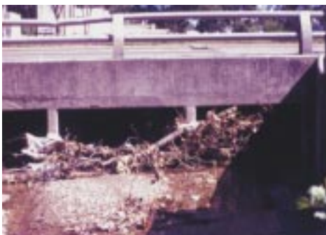
Blocked Storm Channel Culvert
