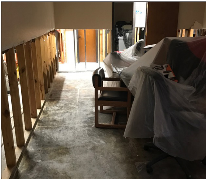
Hurricane Harvey flood damage at one of the TDCJ parole offices.
