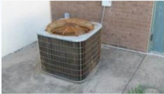
RUSTED AIR CONDITIONER
