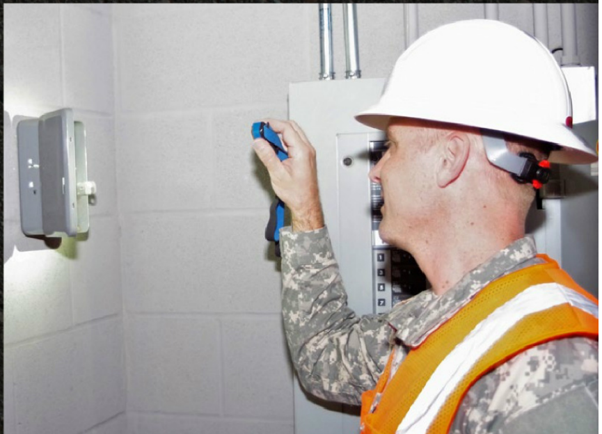
Texas State Guard Engineer Group member Capt. Ian Taylor inspects an electrical circuit box during an installation status report inspection at Camp Swift, Bastrop, Texas, April 2018. (Texas State Guard Photo By: Sgt. 1st Class Malcolm Cowdin)
