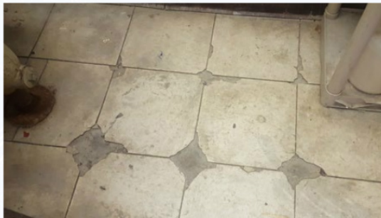
WORN OUT FLOORING
