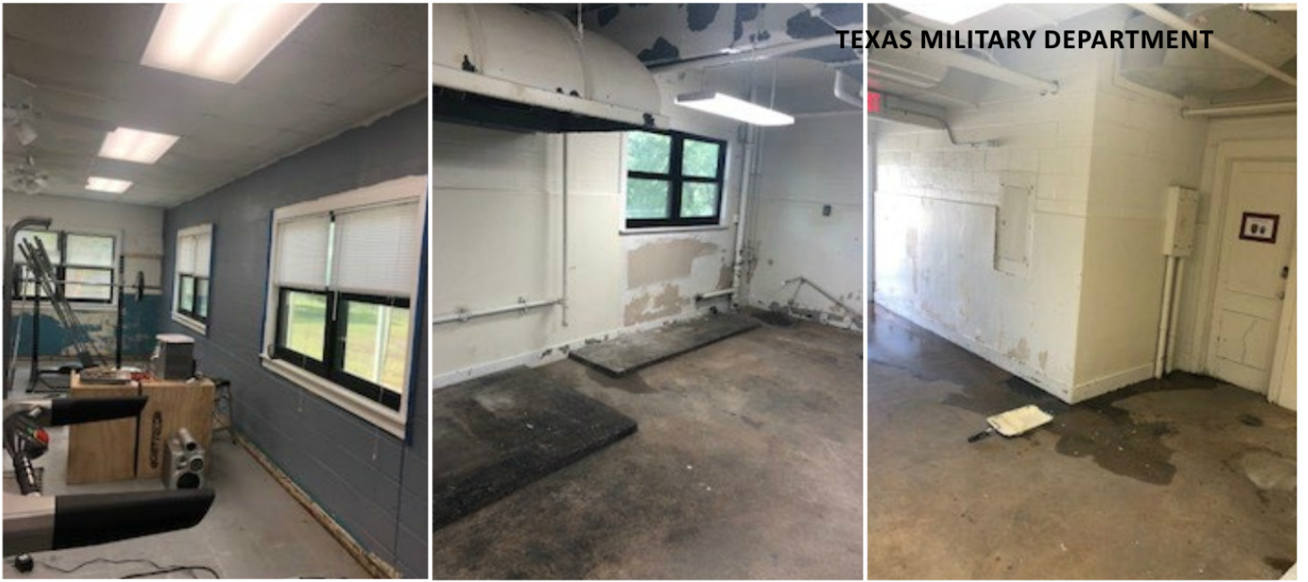
(ABOVE) Collection of photos of the Bee Caves Armory gym before revitalization.
