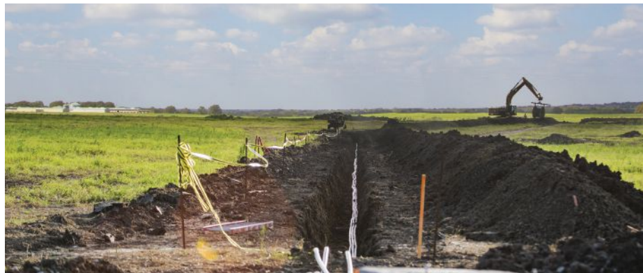
Construction is underway on a several thousand-acre solar farm in the rural community of Otto, about 30 miles outside of Waco.
