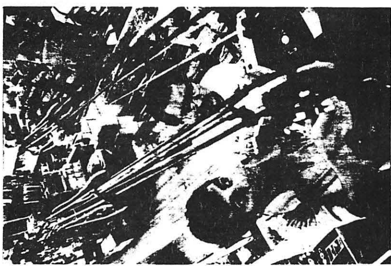
Adrian Dominguez, left, helps Henne Hardware owner Bob Schima with the installation of the three intricate money trolleys on the ceiling of the 131-year-old hardware store. (Photo by Deryl Clark)
