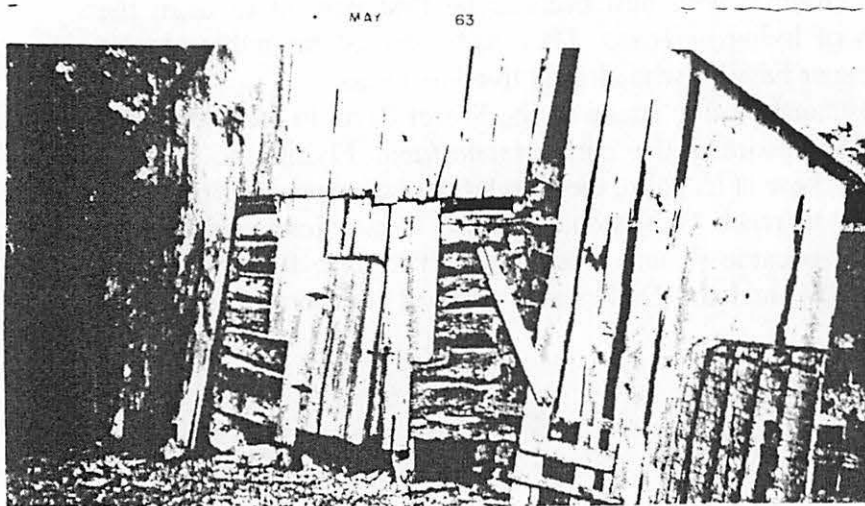
Remains of log cabin built in 1855 by Friedrich Duderstadt. Logs are about 12' x 12' and some 14' long, dovetailed to fit the corners.
