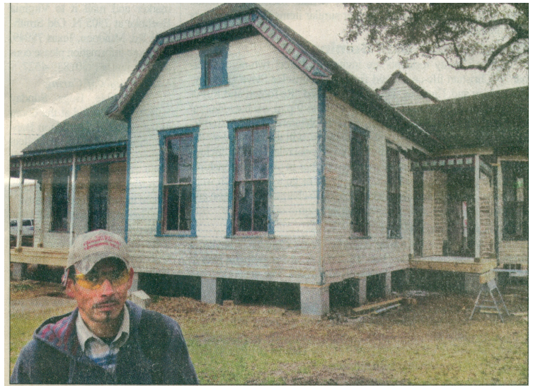
Angel Martinez of Paige is shown here in front of the historic house at 443 N. Washington in downtown La Grange he is helping to renovate, which is set to become a new German themed restaurant with an exterior biergarten.
