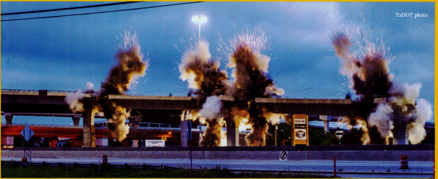
The I-35/U.S. 183 flyover in the Austin District was demolished in May – with some special help!
