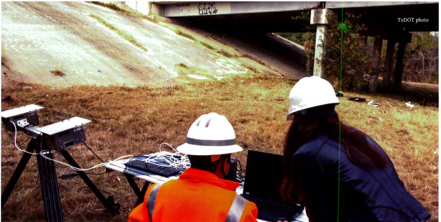
The CIV system cameras are operated by a laptop computer. The system can measure the load-capacity of a bridge with great accuracy.
