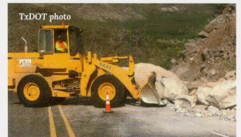
The El Paso District's Special Crew used specialized equipment and a massive loader to move boulders off roads like FM 170 near Lajitas.
