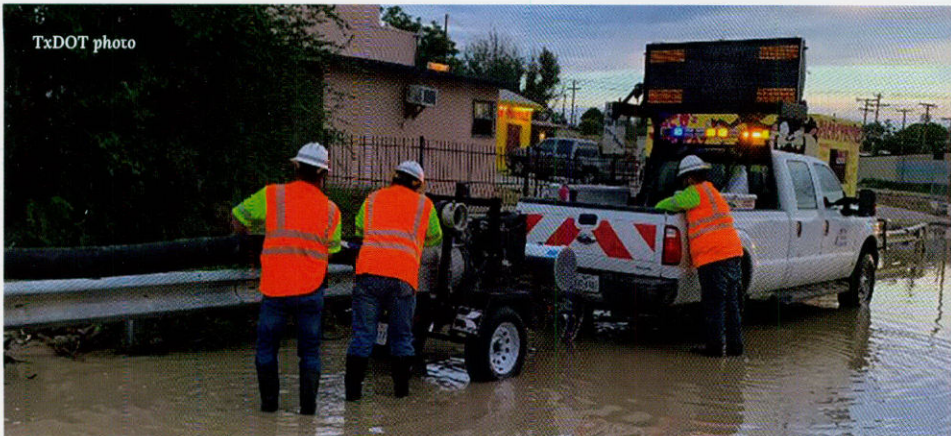
Problem areas kept crews busy around the clock during the storm. Here crews work to clear a flooded section of Doniphan Drive.
