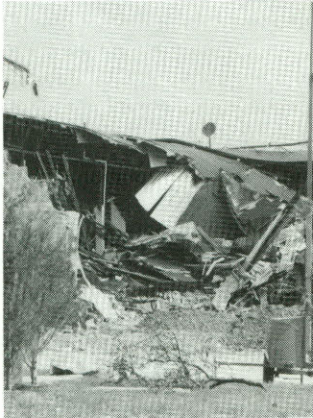
The Albertson's roof in Cedar Park collapsed after being struck by a tornado.
