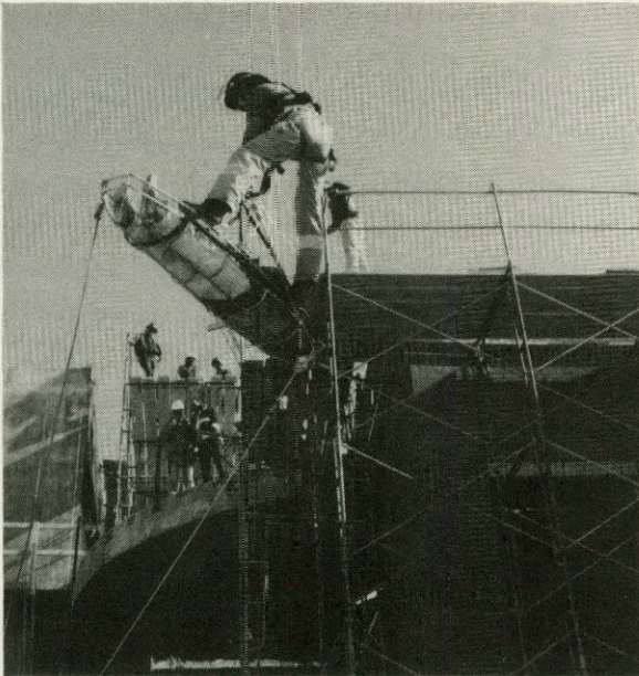
Driver/EMT David Wike of the San Angelo Fire Department attends the victim of a construction mishap as he is lowered to a waiting ambulance. Photo: Ron Perry
