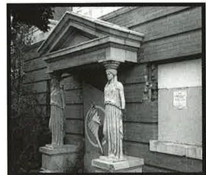
These caryatids at the 1914 Nueces County Courthouse have been neglected for more than 20 years. Because of a deed restriction held by the THC, the building is still standing and has received Round II funding.
