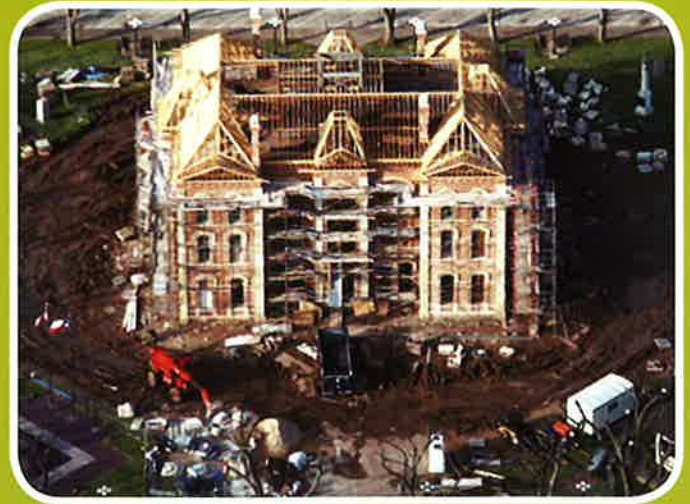
The restoration included the demolition of the 1940s additions and replicating the pressed metal shingle roof and clock tower.
