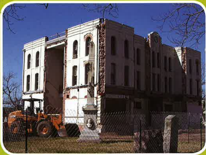
A stucco exterior, added in 1935, is removed from the 1889 Wharton County Courthouse.
