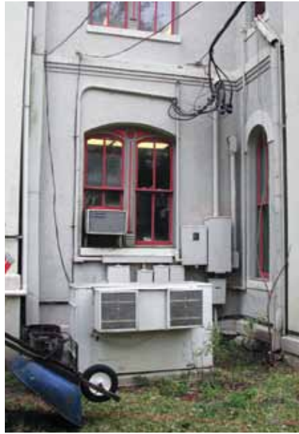
Previously, localized fires have occurred due to aging electrical and mechanical systems in the 1891 Tyler County Courthouse, Woodville
