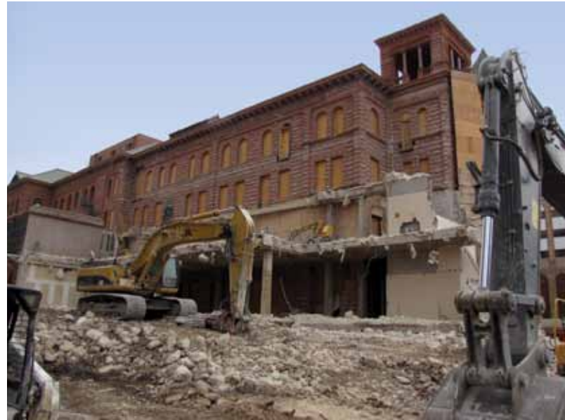
Recent work at the Bexar County Courthouse used demolition robots for efficiency.
