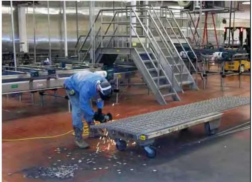
Skinner Baking employee Tyson Keys cuts stainless steel grates, which will be used in the company's revamped facility in Paris. Photo courtesy of J. Skinner Baking
