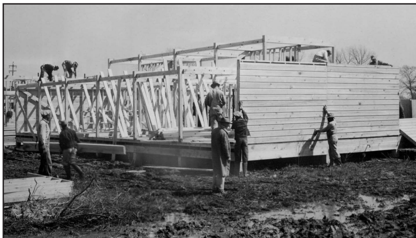
Assembling a housing module at Multimax Village, February 1942. Courtesy of the David Williams Papers, Edith Garland Dupré Library, University of Louisiana at Lafayette.
