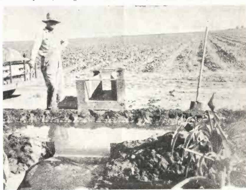
Rectangular Weir and Parshall flume used to measure discharge from the irrigation ditch to the field.
