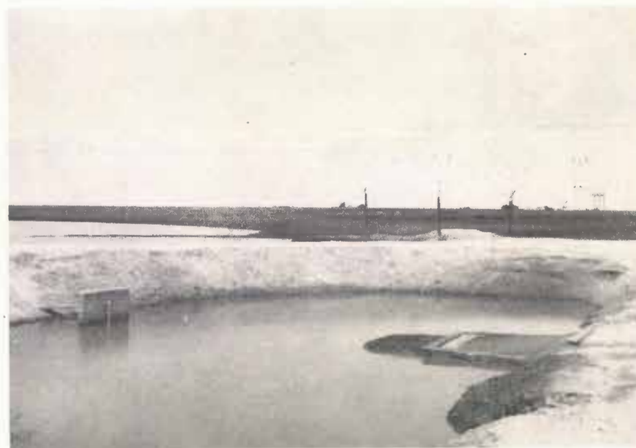
Plate 2—Shows recharge well in pit during recharging experiment.
