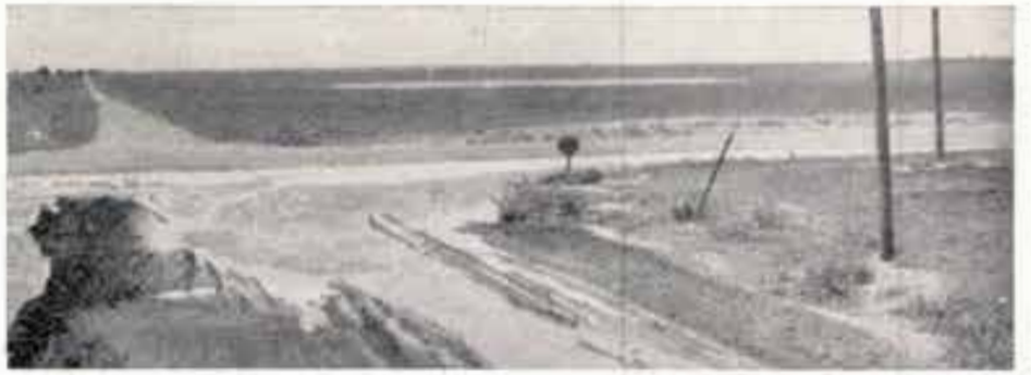
This picture was taken of a county road rendered impassable by water pumped for irrigation. No provision had been made to keep the well water on the farm from which it was produced.
