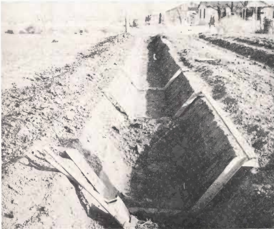
Open ditch being concrete lined to save water that would otherwise be lost to soil seepage. The steep walls of the ditch help cut down evaporation loss.
