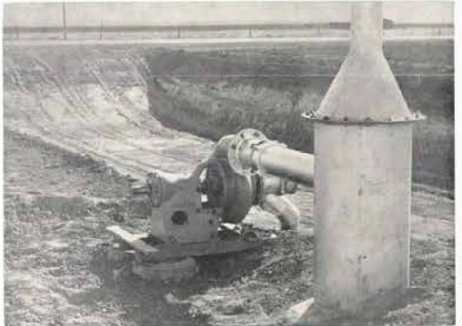
6-inch centrifugal pump picks up "tail-water" from sump and pumps it into concrete pipeline.
