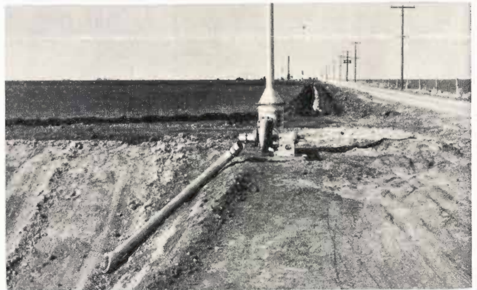
Water enters 12-inch underground pipeline at first riser and is pumped 960 feet up the land to where it joins an existing 15-inch pipeline at second riser.
