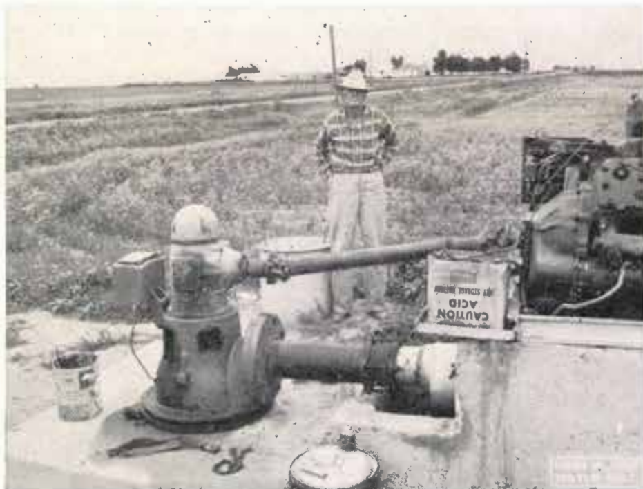
The recharge well pictured above is on land owned by J. A. Howell, about 3 miles west of Idalou. Mr. Howell is standing beside the installation. The 5-inch well is drilled 275 feet deep and cased with 16-inch pipe. The lake, which consists of approximately 10 acres has been drained 5 times this year. On June 17 the lake bottom was dry and ready to plant. About 5 days are required to drain the lake into the well. Mr. Howell normally pumps the well twice a day during the recharging operation for about thirty minutes in order to keep the mud and silt cleaned out of the well.
