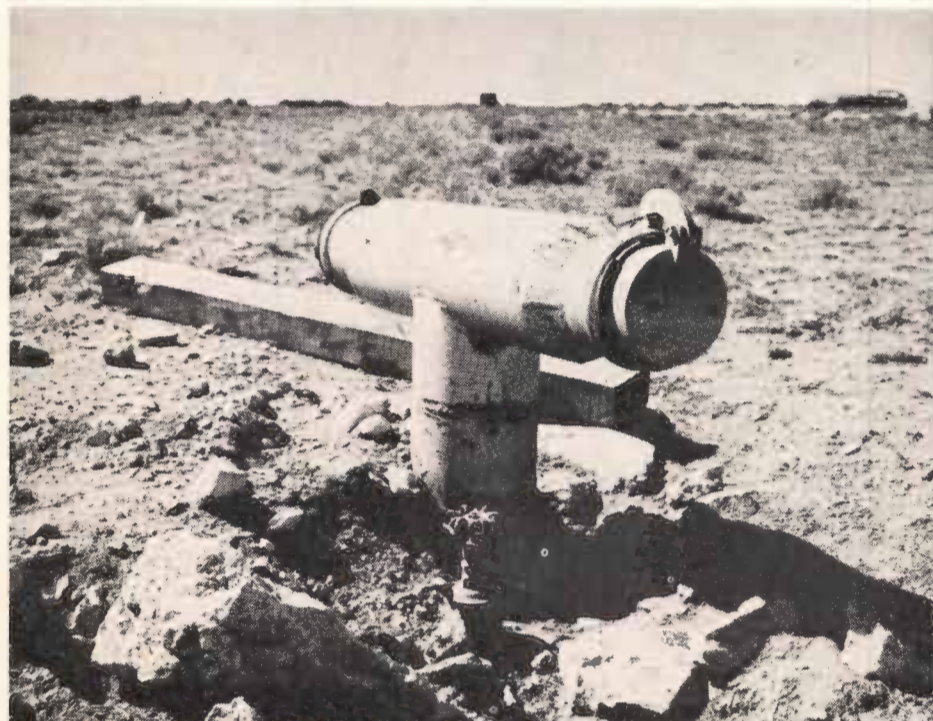
Shown above is a two-way hydrant located at the center of the Wynn farm. 8-inch underground steel pipe carries water to the hydrant from a 460 G.P.M. well. From the hydrant an aluminum surface pipe carries water to the sprinkler heads at either side of the farm.
