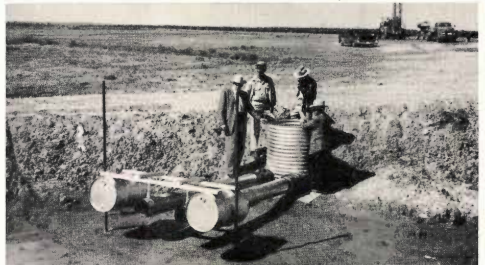
The picture above shows an improved lake intake for a recharge well. The intake pipes are attached to oil drums which will float on the surface of the lake. It has been established that the most silt-free water in a lake is near the surface, consequently, it is believed that this floating intake will allow less clogging matter to drain into the well.
