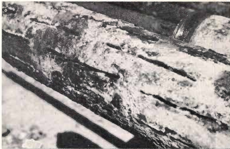
The picture above shows a thick accumulation of algae on the 6-inch strainer which was in the Crew's well below the bowl assembly.
