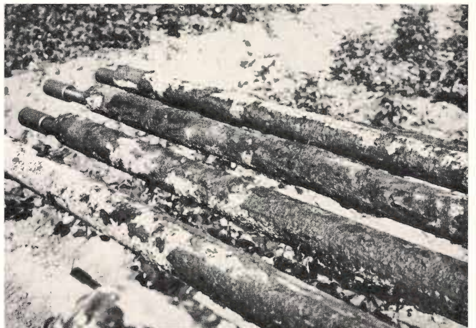
Picture above shows extent of algae growth on pump oil tubing. The oil tubing and inside of column pipe were coated with algae from top to bottom.
