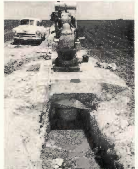
Above is shown a recharge well which experienced a partial cave-in because a packer was not installed.
