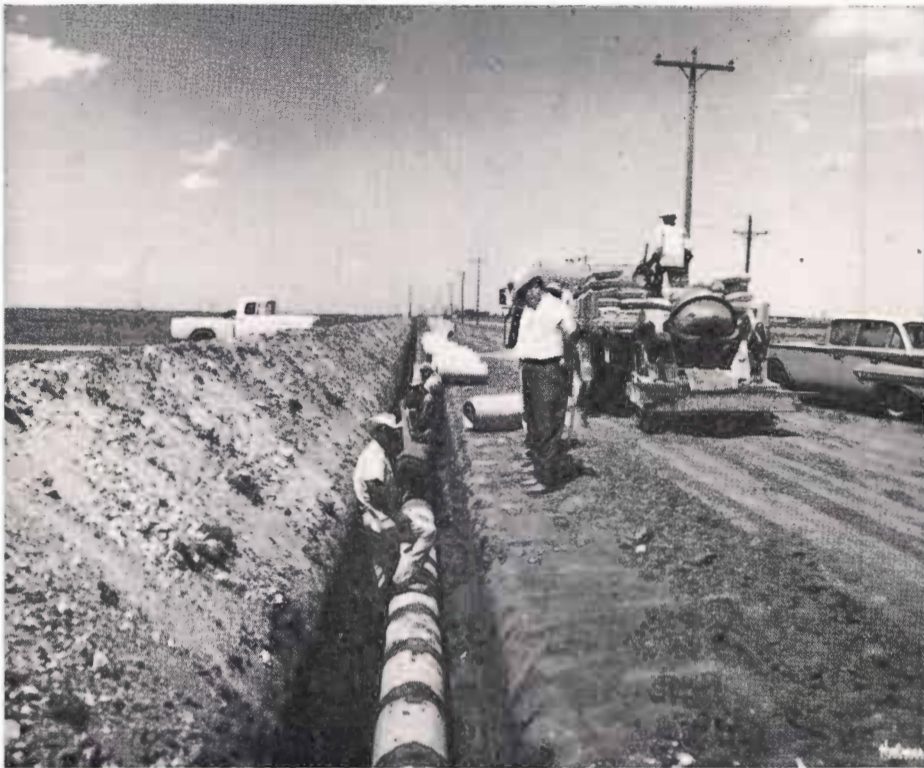
The picture above shows the installation crew putting the finishing touches on the standard mortar-joint concrete pipeline before back-filling with soil. This pipe is in the low-pressure range—about 12 pounds per square inch. Mortar-joint pipelines are the most commonly used in the southern High Plains of Texas.
