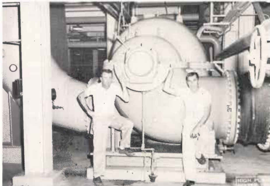
The station is equipped with 6 centrifugal pumps like the one shown above. They circulate 200,000 gallons of water per minute through three steam condensers. Mr. May and Mr. Mixon pose to show comparative size of pump.
