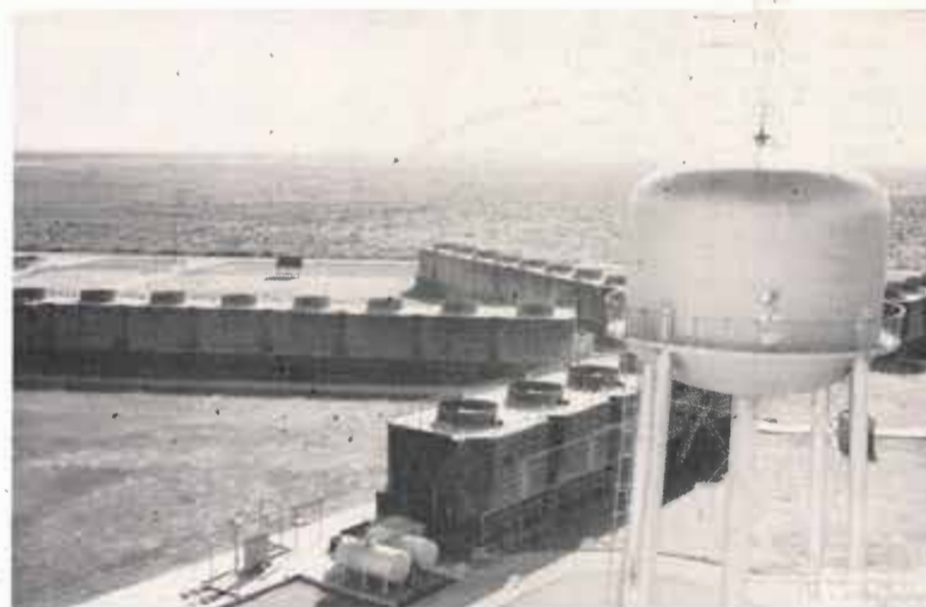
Water that circulates through the steam condensers is cooled by evaporation in the cooling towers shown above. The station has six cooling towers that consist of 46 cells. Each cell is equipped with a large fan that pulls air from the bottom to the top of the cell.
