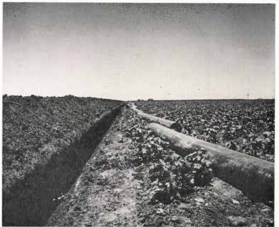
This photograph shows plastic pipe laying near the ditch into which it is to be installed. The pipe comes in 30-foot lengths and it put together by using plastic couplings secured with steel clamps. This pipe is in the medium-pressure class—about 20 pounds per square inch. An underground steel pipeline and an underground aluminum pipeline have also been installed on the new experiment station.
