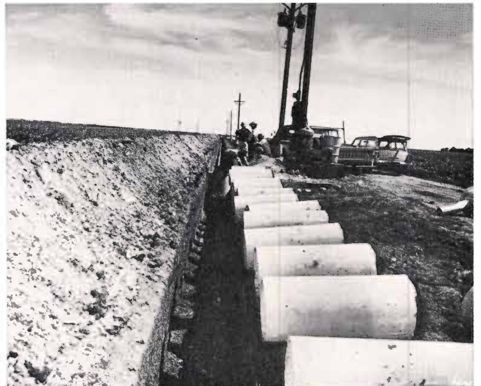
The ditch has been dug and the rubber-gasket concrete pipe is lined up awaiting installation. This pipe is also in the medium-pressure class—about 20 pounds per square inch.
