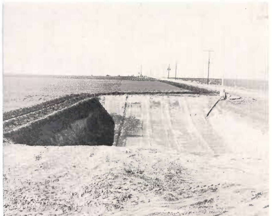
This sump was dug on the Trautman farm west of Hereford, in Deaf Smith County, to catch irrigation "tail-water". The idea is to dig the sump at the lower corner of the farm and channel all "tail-water" into it. Then, by using a centrifugal pump, the water can be returned to a higher point on the farm where it can be used. The Trautmans are primarily vegetable farmers.
