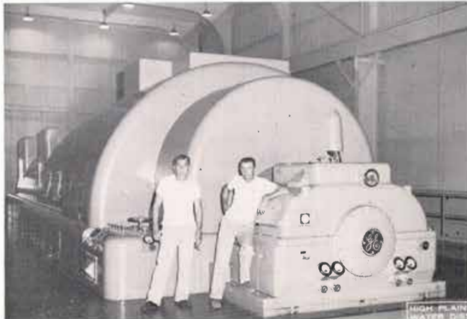
The steam-turbine generator shown above is capable of producing 112,500 kilowatt hours of electricity per hour. The two operators are, left to right, Charles J. Mixon and Harold K. May.
