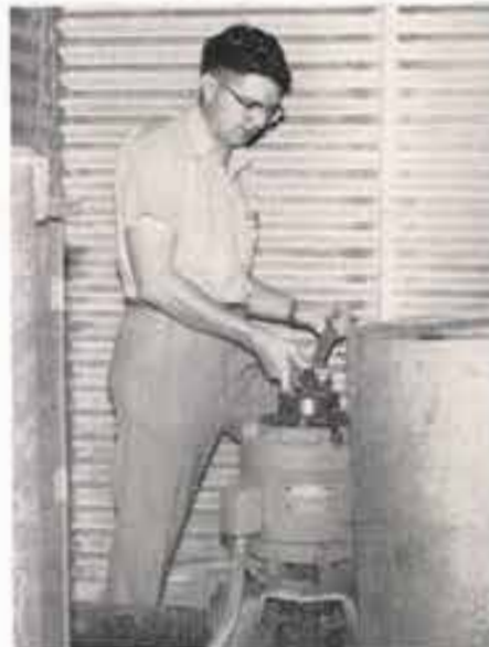
Mr. Schwiesow is shown above as he adjusts the impellers on one of the irrigation wells on the Texas Tech farms.
