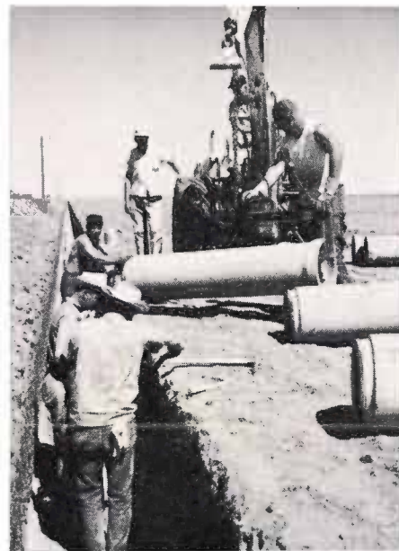
A crew prepares to install a joint of rubber-gasket concrete pipe. This pipe is designed for medium water pressures—in the 20 pounds per square inch range.
