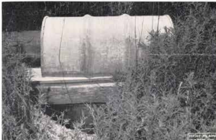
The abandoned well shown above is located adjacent to a Floyd County home where children frequently play. The well is closed improperly. Surface water can enter the well making it a source of contamination. Also, curious children could easily fall into the well. If you have an abandoned well on your property make sure that it is not a source of pollution nor a death-trap.
