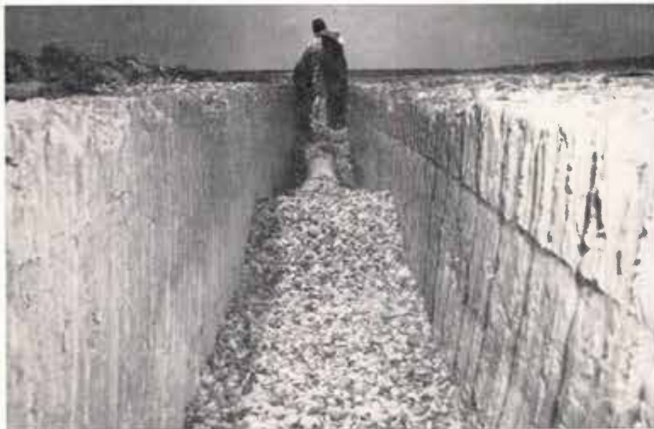
Figure 4 To prevent overlying pea gravel from passing through the openings in the shutter screen, larger-sized gravel was used to form an envelope around the pipe.
