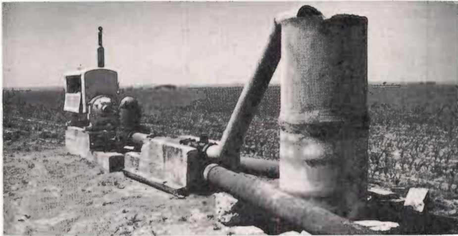
The Newton's have one good 8-inch irrigation well on their 80-acre tract. Note the flow-meter installed on the discharge pipe of the pump. The meter records the amount of well water produced for irrigation.
