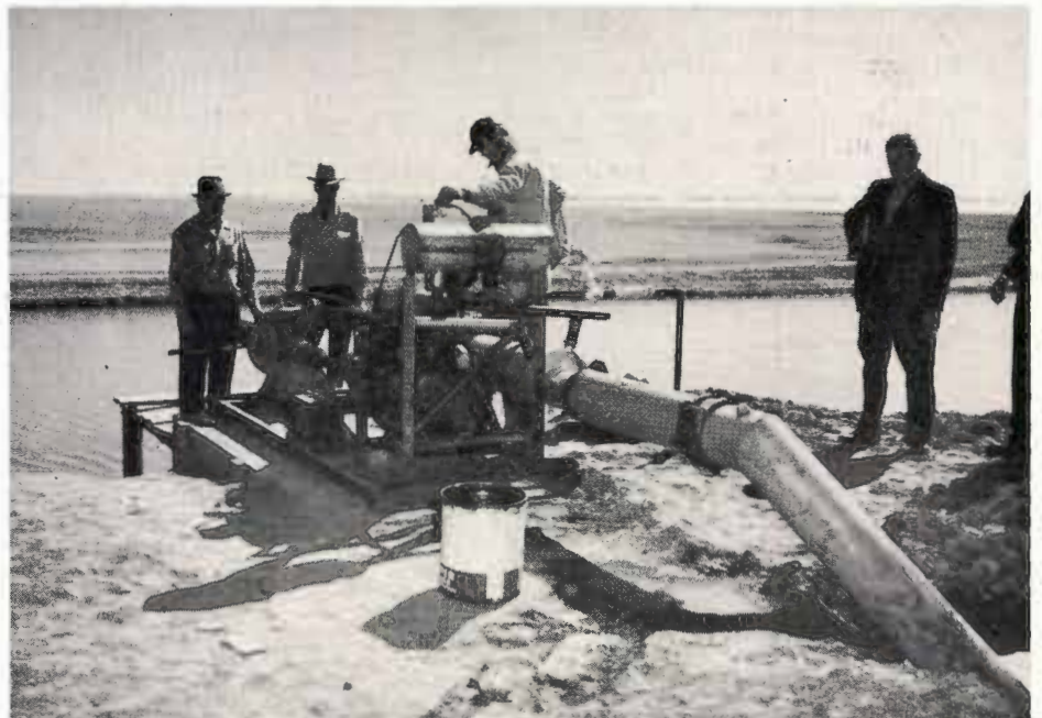
The recirculating pump sends water to any desired point on the Carnahan farm through an underground pipeline system.
