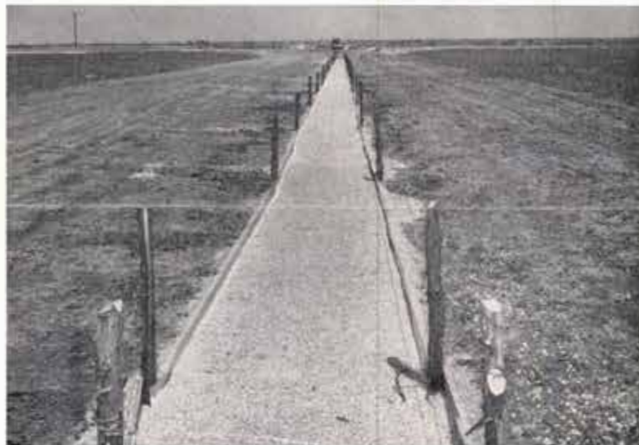
The completed gravel-filter system is shown above. Pea-sized gravel was used to back-fill the buried perforated pipeline. When rainfall runoff enters the lake it will submerge the pipeline. As the valve is opened to the recharge well the muddy lake water will filter down through the gravel to the pipeline. The filtered water will then move by gravity into the well.
