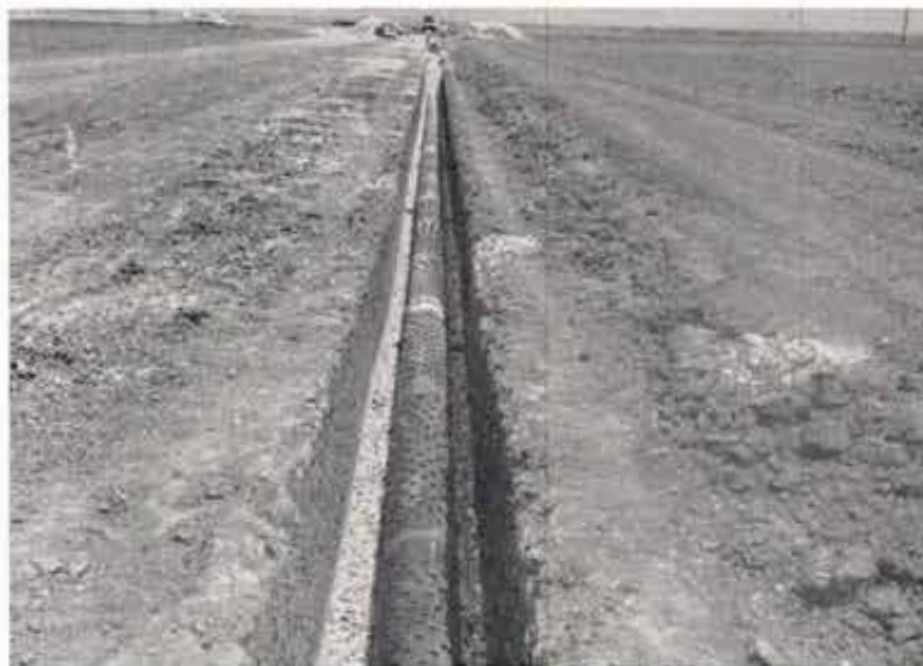
A ditch was dug from the recharge well out into the dry lake bed. Sixteen-inch steel shutter-screen type casing was laid in the ditch. The steel pipe was underlain by a 6-inch thick gravel bed.
