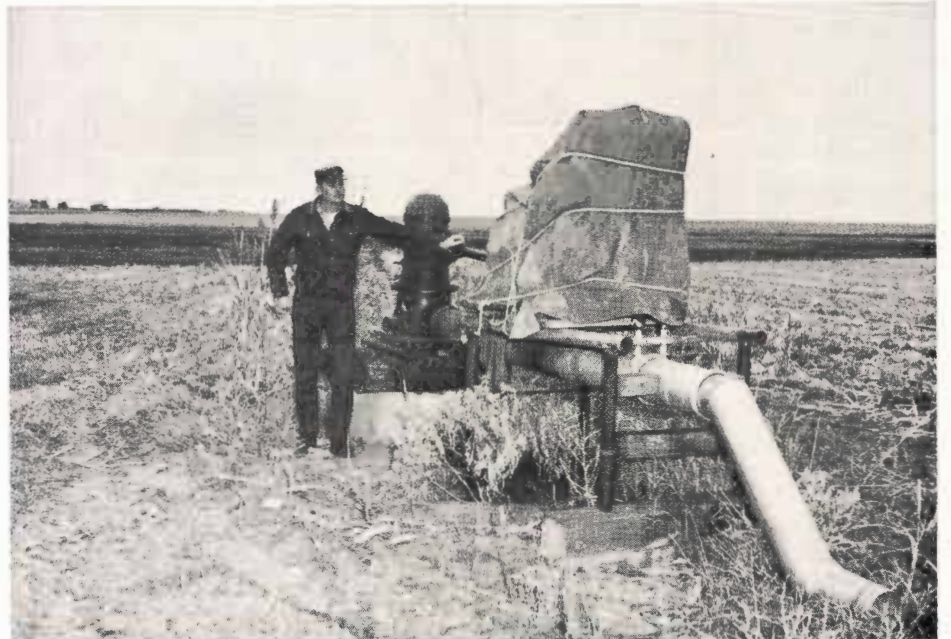
Mr. Falkenburg is shown along side the lake pump. The pump is set in a concrete sump, 30 inches in diameter and 13 feet deep. The pump consists of a standard 2-stage 10-inch bowl assembly, 10 feet of 8-inch column pipe, an 8-inch discharge head and a 1 to 1 ratio gearhead. An automotive engine powers the pump. The discharge pipe of the pump is attached to the farms' underground concrete pipeline system.
