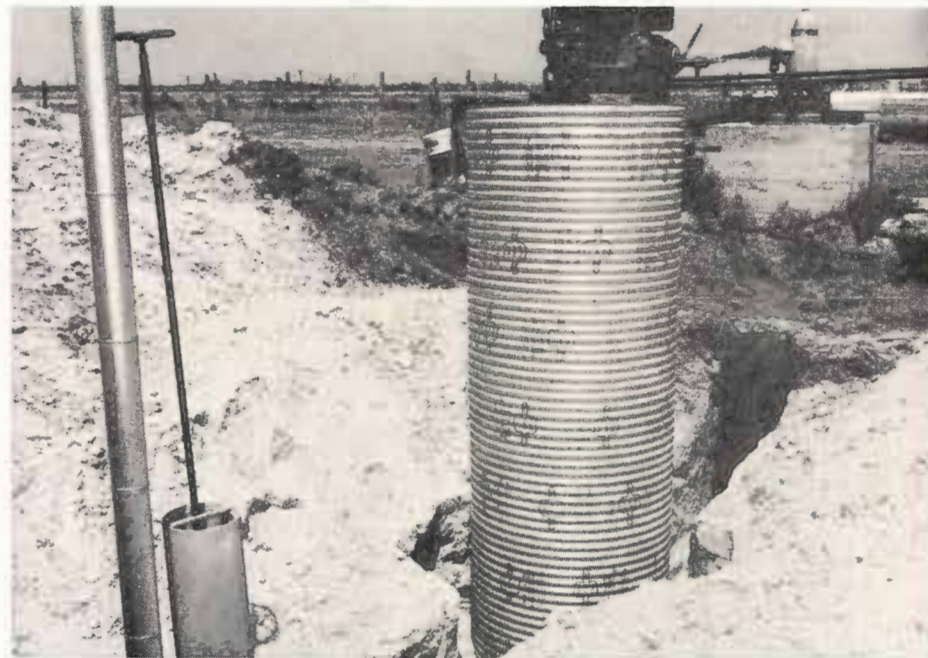
Figure 6 Shown above, left to right, is an air vent, a 12-inch valve extension and a 60-inch steel culvert. The culvert affords an access to a meter and an 8-inch valve.
