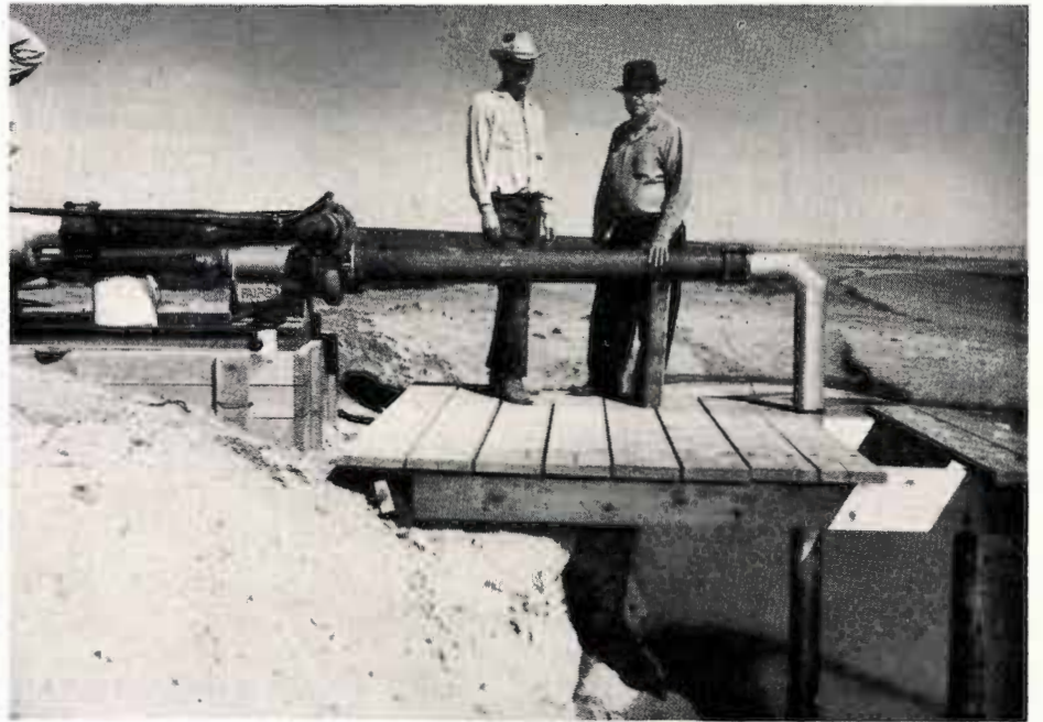
Tommy Carnahan and his father, C. D., stand beside the suction pipe of their 6-inch centrifugal pump. The pump is primed automatically and produces approximately 1000 gallons of water per minute.
