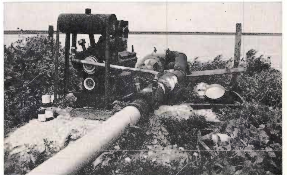
Steve Clements of Deaf Smith County installed the 6-inch centrifugal pump and engine shown above near the edge of a rather large lake on his farm located northwest of Hereford. The High Plains Water District attached a flow-meter to the pump's discharge line in order to calculate the amount of water salvaged from the lake. Since March of this year, Clements has reclaimed water from the lake for irrigation valued at more than $8000.
