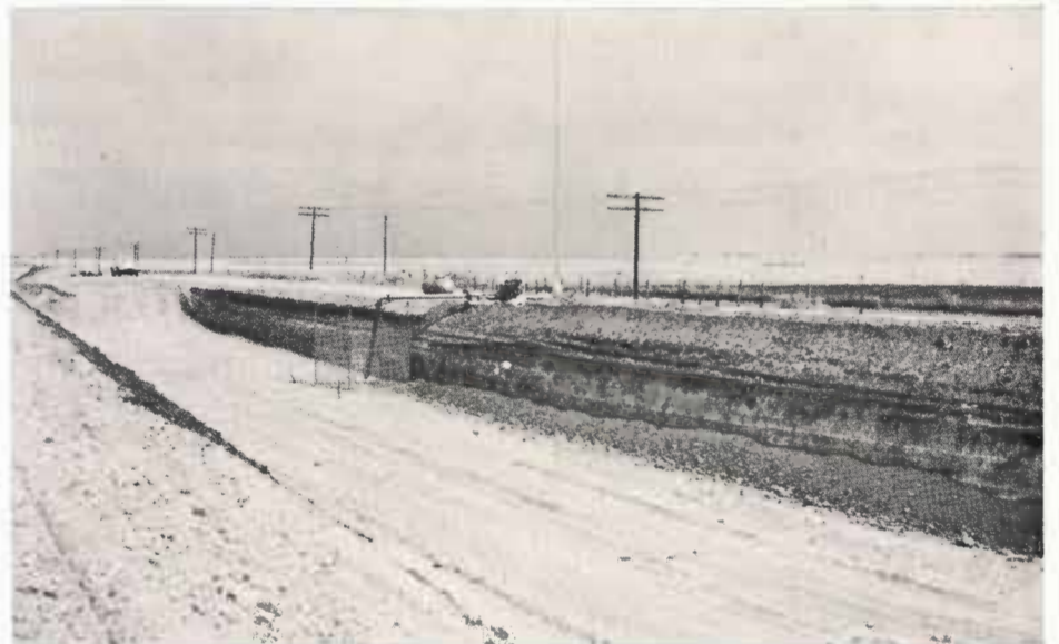
Godwin's re-circulating pit is 40 feet wide, 330 feet long and 10 feet deep. It is located in the southeast corner of the farm (the lowest point on the farm) so irrigation "tailwater" can gravity flow into the pit from the cropland.
