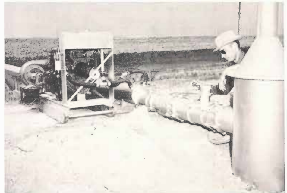
A flow-meter was temporarily installed in the discharge line of the re-circulation pump by the High Plains Underground Water Conservation District. It will be used to calculate the amount of irrigation "tailwater" salvaged and pumped back to the cropland through the system. Godwin records the reading on the meter prior to turning "tailwater" into the pit.
