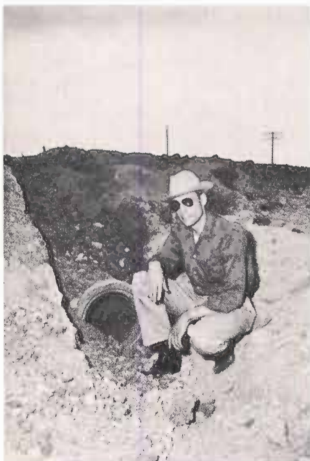
Irrigation "tailwater" from neighboring land will be diverted from the road bar-ditches to the re-circulating pit through two concrete pipes. Godwin is shown as he kneels near the inlet of one of the intake pipes.
