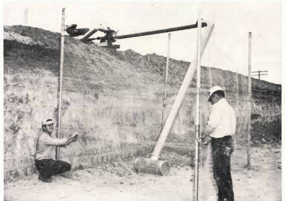
Harley Bryant and Douglas Ross, employees on the Godwin farm, are shown as they install a wire trash guard around the suction intake of the re-circulation pump. The wire guard will keep any large debris from entering and perhaps damaging the pump.
