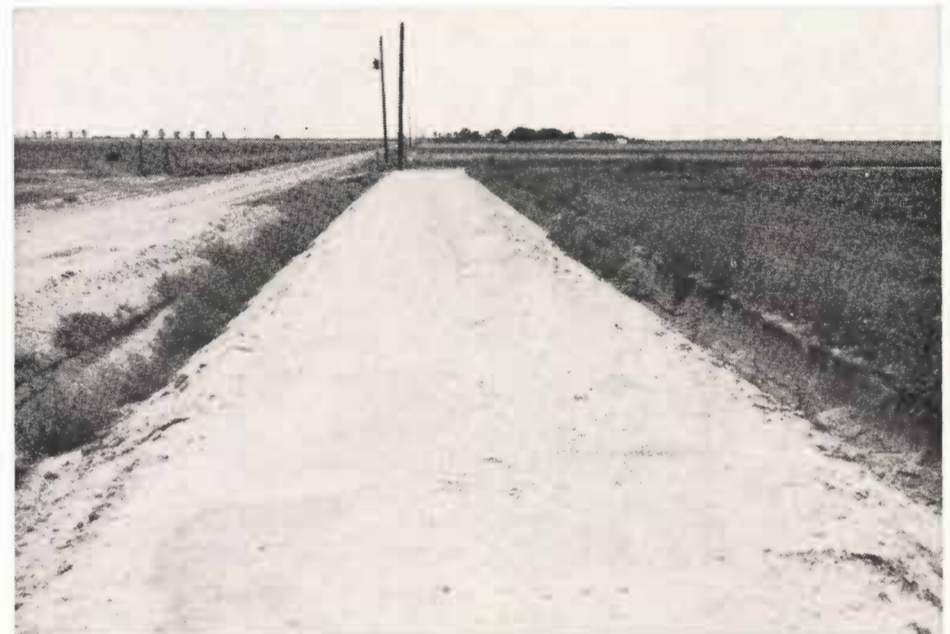
Notice the long low pile of soil removed when the ditch was constructed. The soil can easily be replaced if the ditch is ever abandoned.
