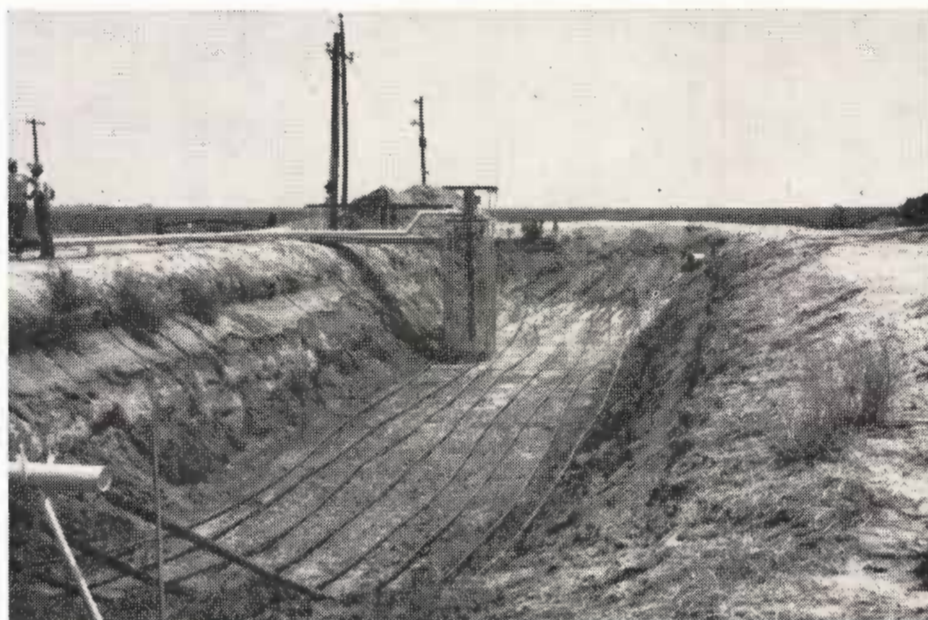
A "birdseye" view of the Menefee installation. Plastic pipes on the floor of the pit carry water for agitation of silt.
