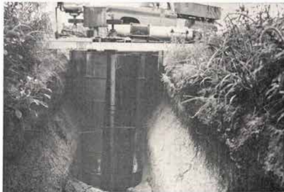
Tailwater pump and ditch located on the Spencer Hough farm in Parmer County. Hale County visitors viewed this installation with interest.
