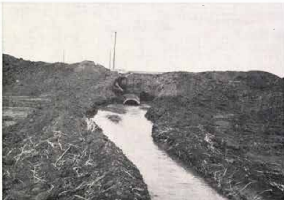
Water flowing from Godwin's pit is cut down to eliminate breaking his irrigation ditch. This water could be running down the bar ditch and wasted.
