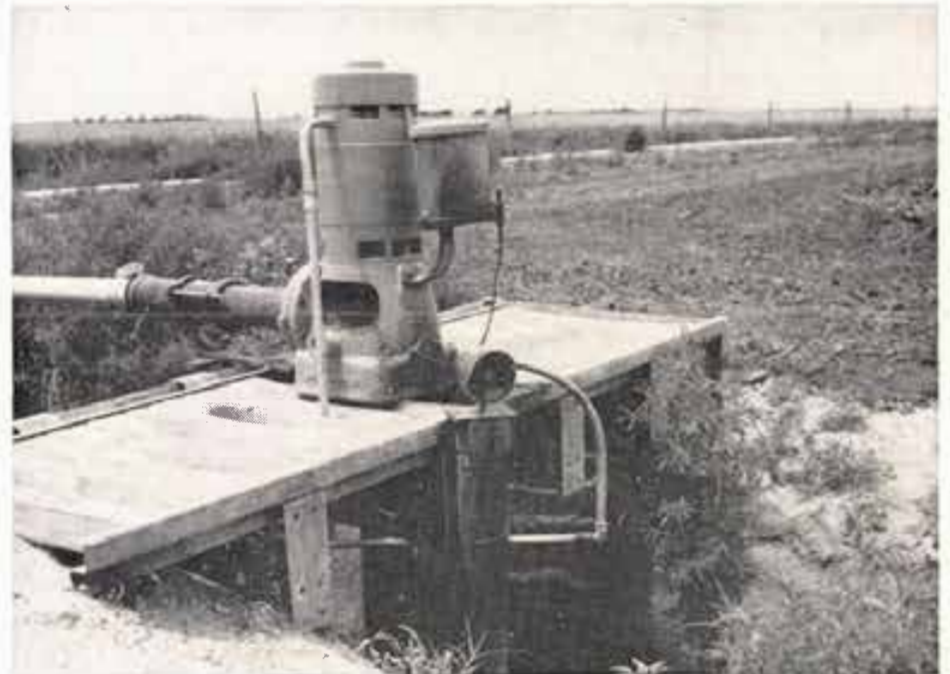
A Close up view of the vertical turbine pump and the three horsepower electric motor used to lift the water from the ditch. In the foreground is the electric switch, connected to a float, which turns the motor on and off.
