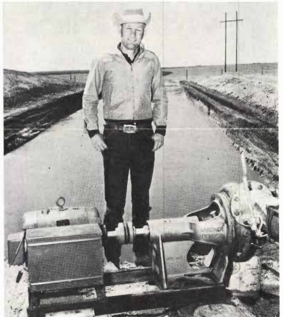
This tailwater installation system is located on the Jack Dunn farm, operated by Mr. J. D. Kirkpatrick. The farm is located about 2 miles west of Bovina, Texas. This system was installed in 1963. The pit was constructed 150 feet in length, 50 feet wide and 15 feet deep with a capacity of almost 700,000 gallons. Kirkpatrick installed a 4" centrifugal pump with a maximum capacity of about 700 gallons per minute, powered by a 7-1/2 hp electric motor. Only a few feet of underground pipeline was required to tie this installation into an already existing system. The system cost about $2000 to install. The High Plains Underground Water Conservation District assembled records on the amount of tailwater pumped by this system. In 1963, Mr. Kirkpatrick recovered a total of 53 acre feet of water. In 1964, 158 acre feet of water; 1965, 103 acre feet of water; and in 1966, 113 acre feet of water for a total of 428 acre feet of water. An average of about 105 acre feet per year.
