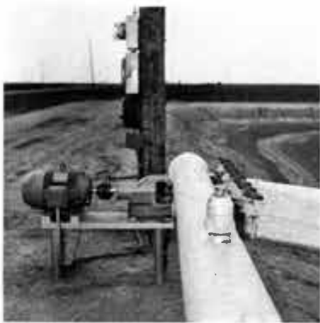
Control facilities, motor and centrifugal pump and valves used to regulate flow through the silt suspension return flow pipes (eight in number) pump and control facilities are located atop a 2-ft by 20-ft. wide berm that surrounds the 180-ft by 180-ft by 12-ft deep pit.
