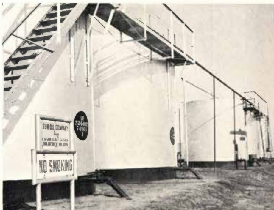
Sun Oil Company tank batteries.
