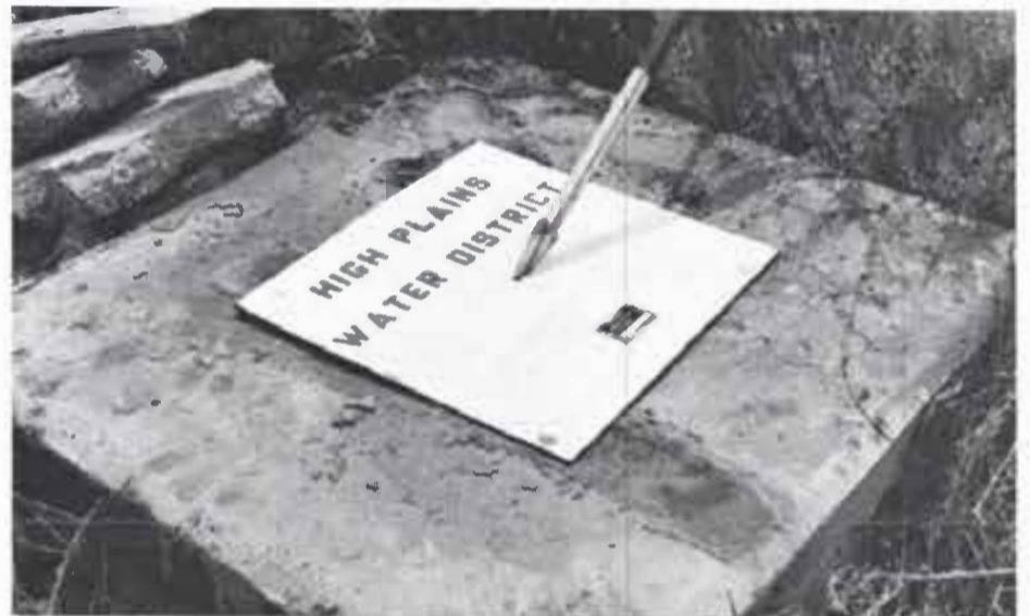
Shown in this photo is the same well that can be seen in the photo at the top of this page. It has been capped in such a way that it is no longer a danger. The heavy steel plate has a pipe welded below it which is inserted into the well, thus preventing accidental or easy removal.
