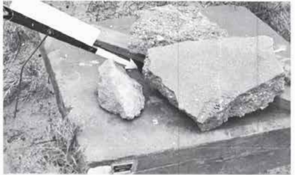
The observation well shown above was improperly covered as may be seen before it was properly capped. Wells which are uncovered or improperly covered as this one should be corrected by closing and capping the well in an approved manner.
