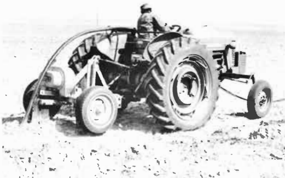
The tractor above is pictured as it lays the underground pipe for a subirrigation system. The pipe rests above the ground in front of the tractor and is fed into the narrow trench being dug by a vibrating plow. (Photos by Tony Schertz)
