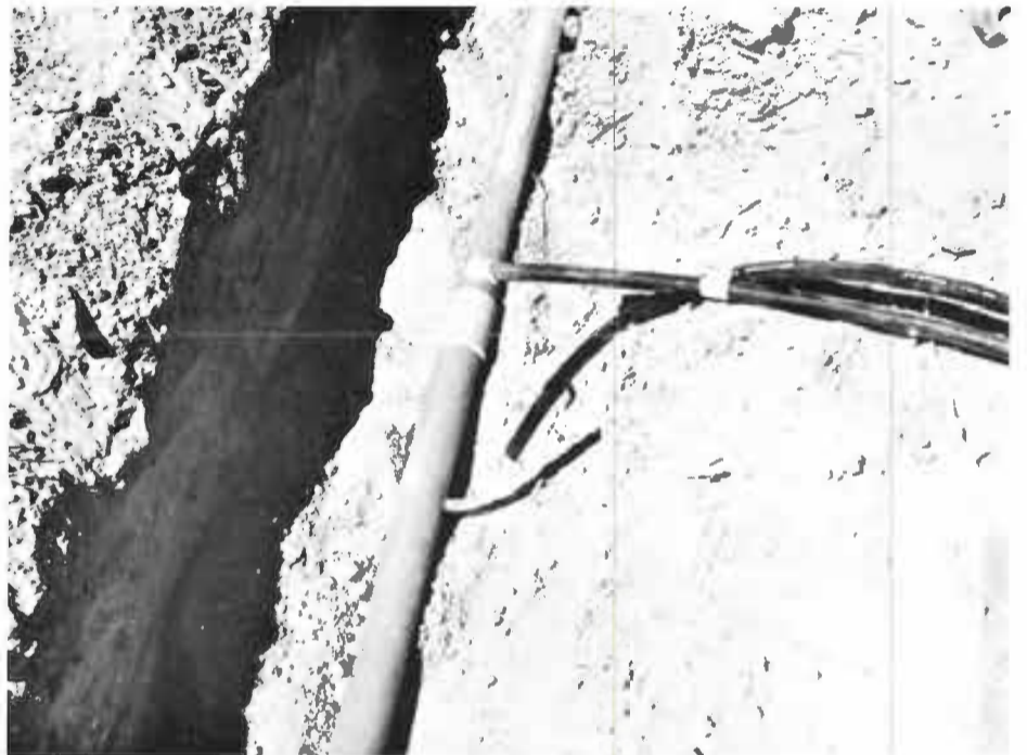
The smaller plastic pipe on the right is the one supplying water to the system's orifices, which are placed at the required intervals. The larger pipe on the left, to which the smaller pipes are attached, are the header pipes.
