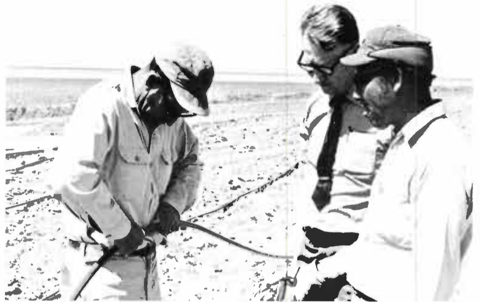
Shown above coupling the flexible plastic pipe before it is laid underground is Blez Gutierrez. Watching are Dale Brown and Luis Arguello, both of Lubbock. This system was being installed on a farm close to Lubbock.
