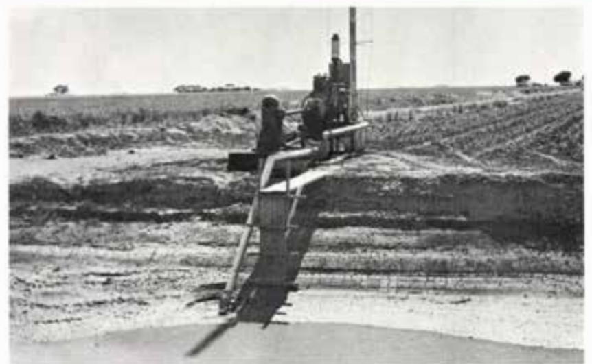
need for additional underground pipeline for the tailwater return system. This tailwater pit is located in the ditch (enlarged) along a turnrow separating two farms. This irrigator can also divert water from the road ditch (to the left of the right-hand photograph) into his tailwater pit. Is this innovating farmer making money with the water escaping from your farm?
