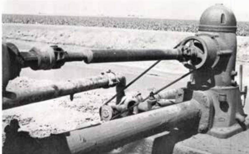
Planning and innovation are the keys to economic tailwater reclamation. This unique tailwater return system employs a small centrifugal pump belt driven from the well's drive shaft. A small pipe with a valve connected to the well pump discharge line supplies water for priming the tailwater pump. The tailwater is pumped directly into the underground distribution system at the well site. The location of this well at the low point on this farm eliminates the
