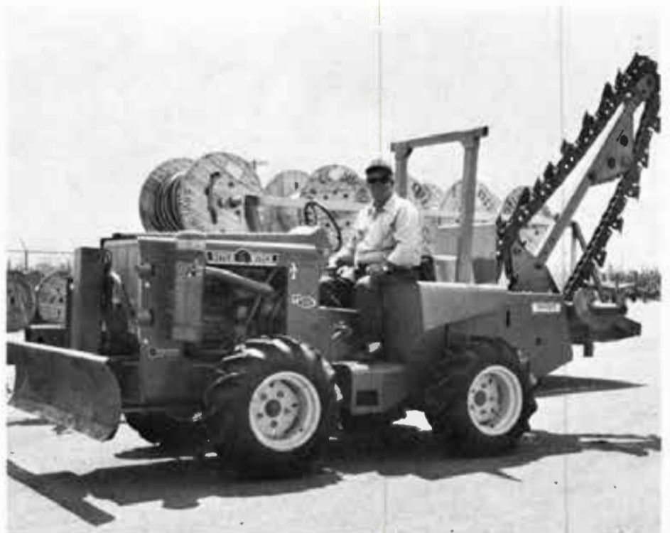
The special equipment shown in this picture is used to bury electrical cable serving sprinkler systems.
