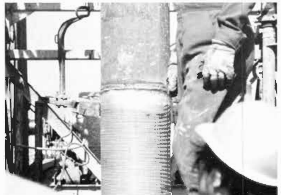
The Johnson (commercial) well screen being installed in the new Halfway Station irrigation well by High Plains Drilling Incorporated.
