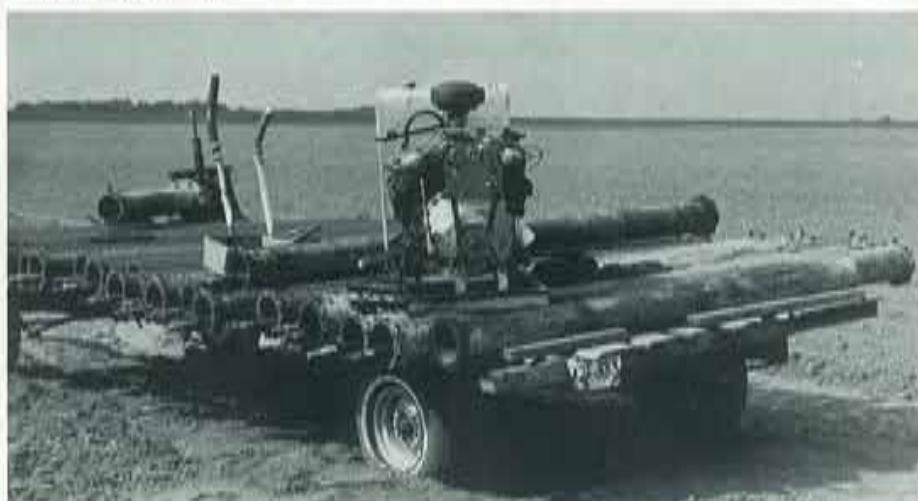
Pump and motor removed from the Lewis Cox and Son well, April 1977.
