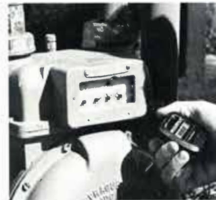
Natural Gas Meter
