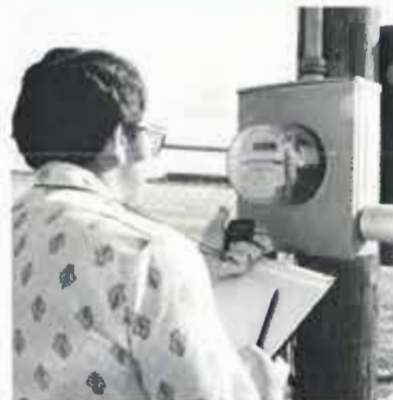
Watt Hour Meter
