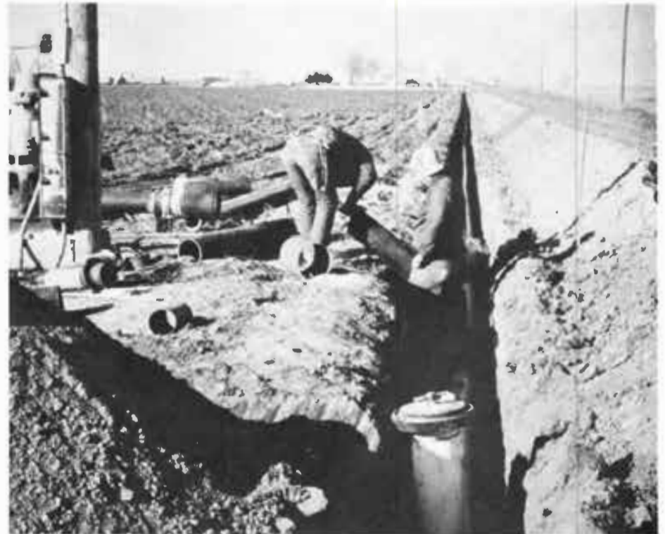
TEN THOUSAND miles of underground irrigation pipeline deliver water to High Plains crops and stop evaporation or deep percolation losses from open ditches.
