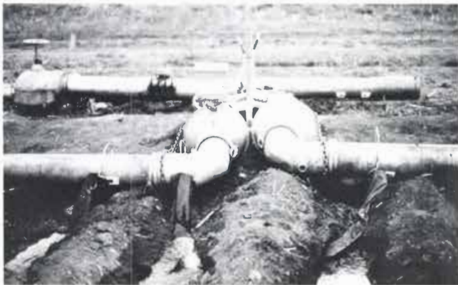
FROM ONE PIPE to another, water is automatically redirected through the diaphragm control valve and a Y shaped connector to gated pipe to furrow irrigate half the rows at set intervals.
