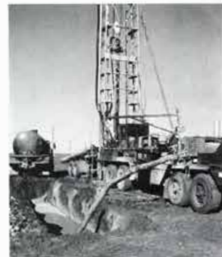
A TYPICAL rotary water well drilling site. This mud pit lacks any barrier to prevent circulation of solids with drilling fluid.
