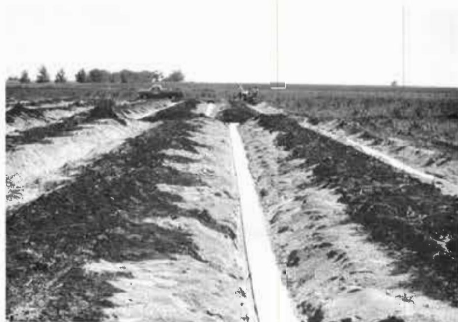
HITEK DRAIN FIELDS —In this 1986 file photo, some of the 19 V-shaped ditches are shown with HiTek filters in place. These filter drain lines are connected with PVC pipe to a central water line entering the recharge well. Tech researchers state the initial flow rate for the combined filtration systems is 200 gallons per minute.
