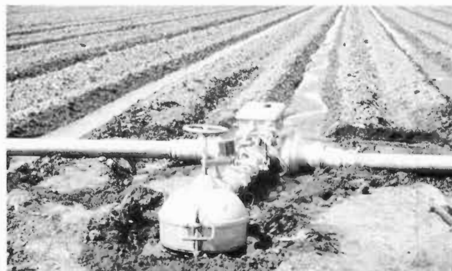
SURGE VALVES USED ACROSS TEXAS — More than 3,000 surge valves are currently used across the Texas High Plains to irrigate cotton, corn and soybeans. Surge irrigation improves furrow irrigation efficiencies by 10 to 40 percent.
