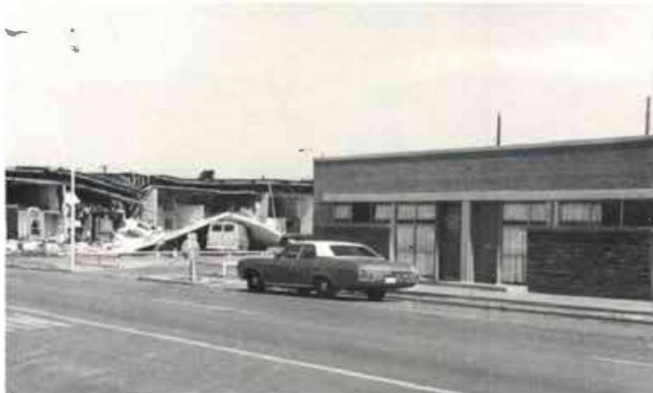
TORNADO DAMAGE — The offices of the High Plains Underground Water Conservation District No. 1 are shown at 1628 15th Street, Lubbock, Texas. Note the building at left that was destroyed by the May 11th storm. The building faces Avenue Q at the 15th Street intersection.
