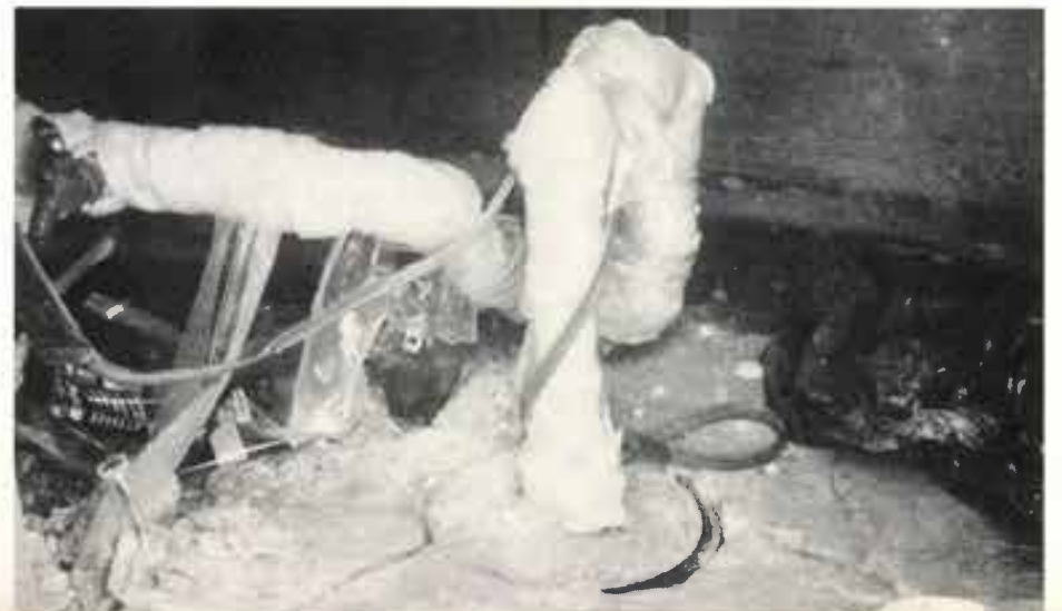
A CONTAMINATED WELL — Contaminants have entered this domestic water well through the cracks in the pump base and openings around the casing. See the October 1987 Cross Section for a review of proper water well completion specifications.
