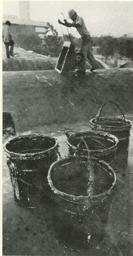
TRIMS's roof rolls like a choppy sea and made a challenging job for these roofers. Above, one worker finds relief from the heat with cold water.
