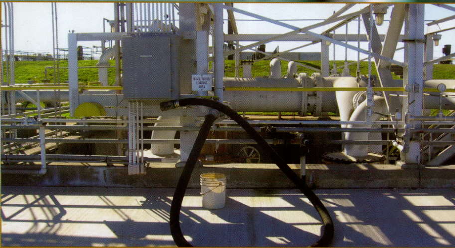
Pumper trucks can pull right up to this loading area at Washburn Tunnel Facility when another treatment facility needs an injection of hard-working micro-organisms.
